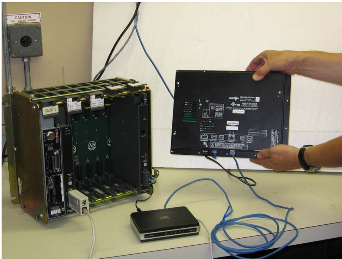
DF1 TCP via Ethernet (shown using PLC Ethernet Module, network switch and KING-GAGE LP3 display module)
